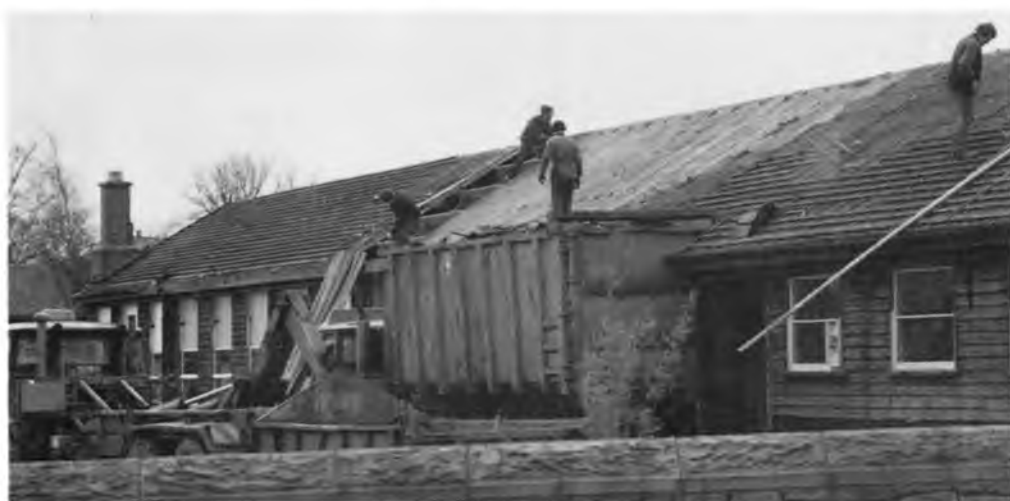
Work begins on demolishing the wooden huts to make way for the pool.
