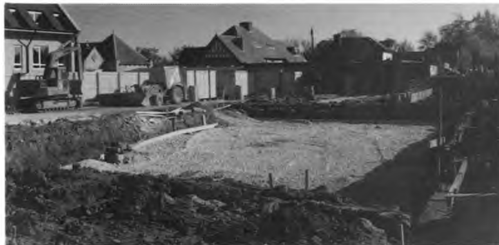
The site of the pool with the new wing, left, and Horncliffe, right.
